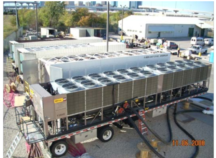
Temporary Chillers Carrying Load During Central Plant Modifications
