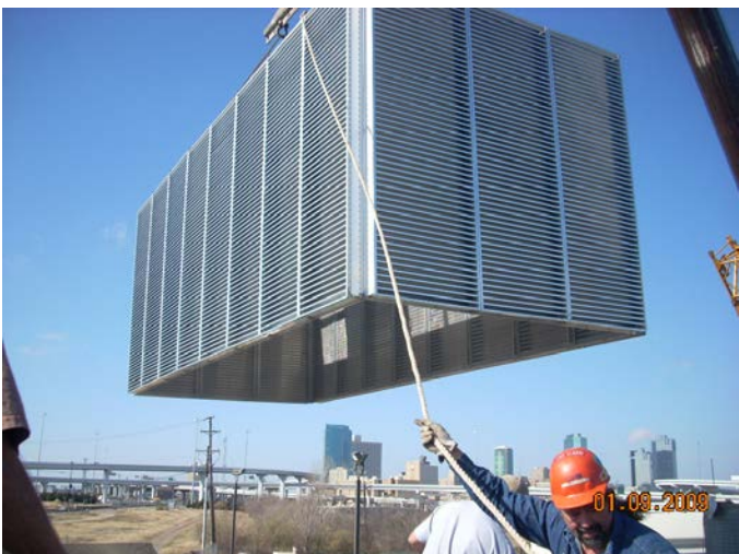
Genset Air Intake Louvered Penthouse
