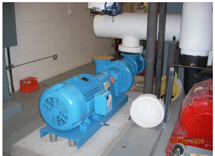
New Chilled Water Pump installed
