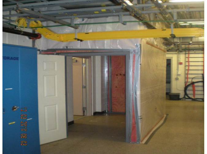
Switch Room Dust Protection Wall
