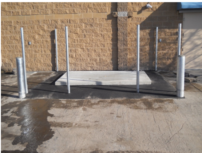
Concrete pad for Liebert Condensers
