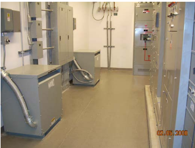
Completed Electrical Gear Installation
