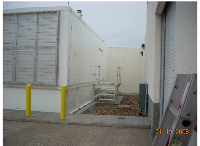
New 1500kW Generator with Enclosure
