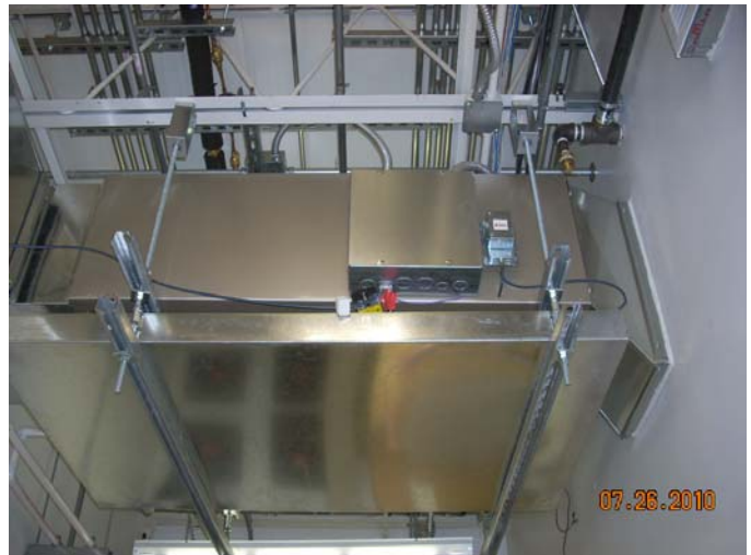
New Ductwork above Live Switch
