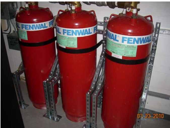
New Seismic Bracing at FM 200 canisters
