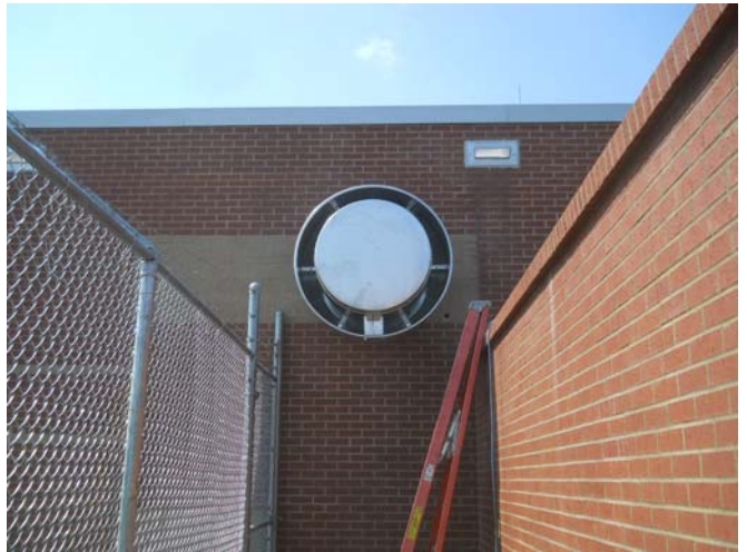
Exhaust Fan Installed
