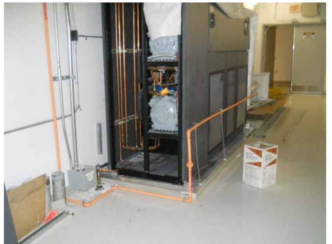
VESDA Piping Installed
