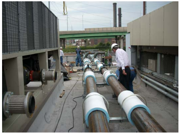
Chilled Water Piping Installation
