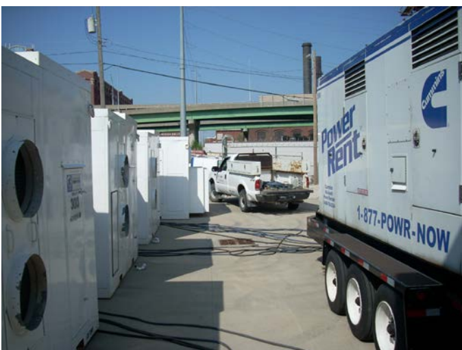
Temporary Cooling Units
