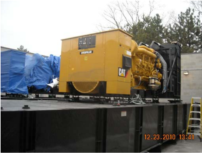
New 1500kW Generators Set
