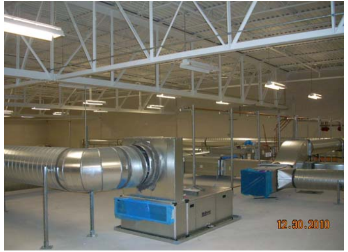
New AHU and OAU and Associated Ductwork
